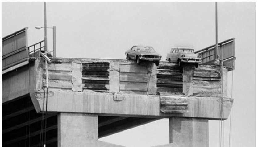
Cars hanging over Hobart's Tasman Bridge in 1975 after a section was knocked down by a ship (photo from ABC)
